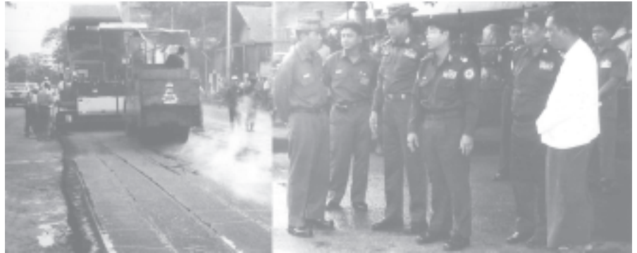
Commander Maj-Gen Myint Swe, Mayor Brig-Gen Aung Thein Lin inspect repaving of Strand Road in Kyimyindine township. — (YA-KA-TA)
