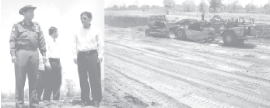
Minister Maj-Gen Htay Oo inspects digging of canal for water supply for Meiktila Lake. — A&I
