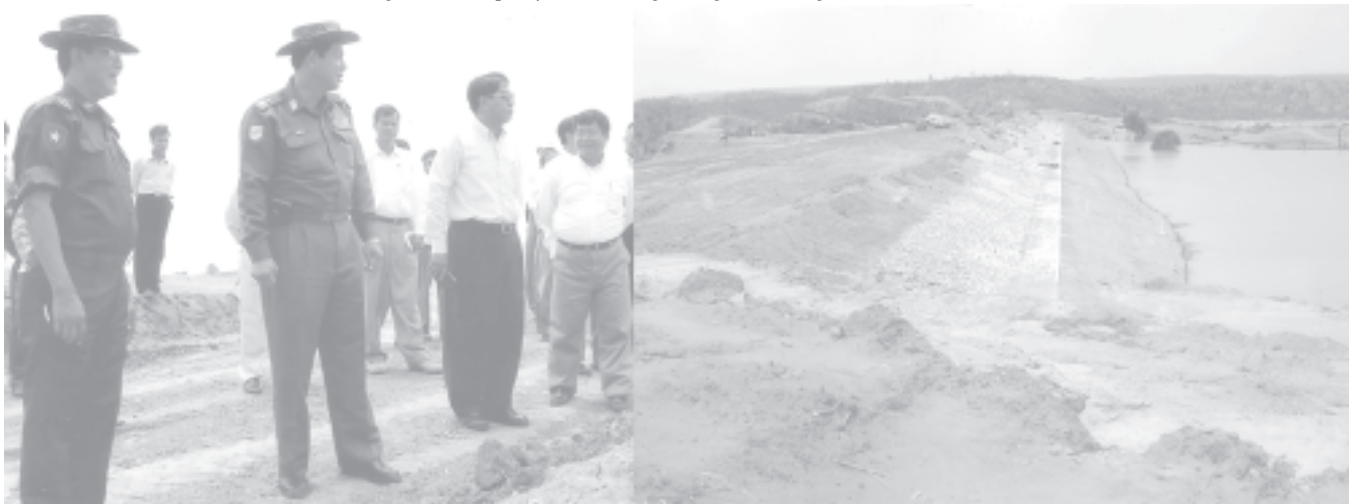
Minister for Agriculture and Irrigation Maj-Gen Htay Oo oversees construction of Myohla (Tatkon) Dam near Inkhon Village of Tatkon Township.—A&I
