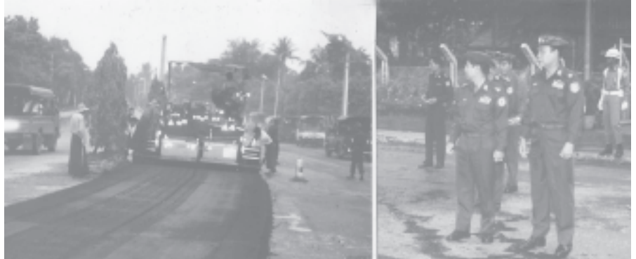
Commander Maj-Gen Myint Swe and Mayor Brig-Gen Aung Thein Lin inspect placing of asphalt concrete on Kyaikwaing Pagoda Road. —YANGON COMMAND
