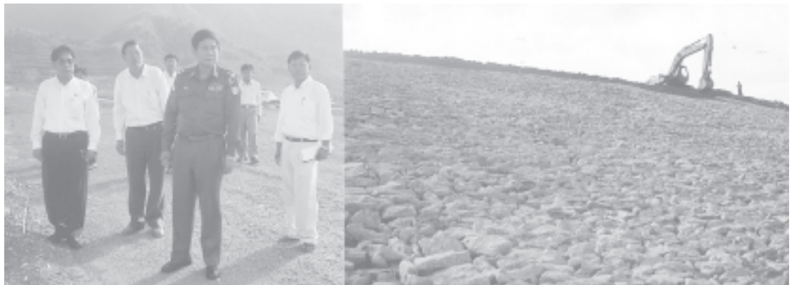
Minister for Agriculture and Irrigation Maj-Gen Htay Oo oversees construction of main embankment at Kataik Dam Project in Paung Township. — A&I
