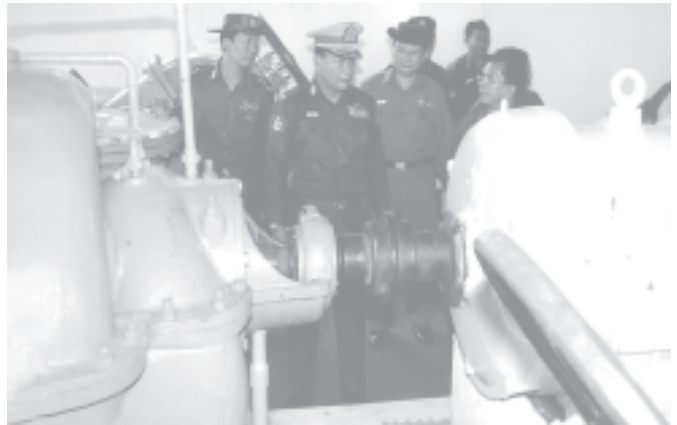
Mayor Brig-Gen Aung Thein Lin inspects Relay Pump (Pyawbwesu) in Hmawby Township. (News on page 2) — YCDC
