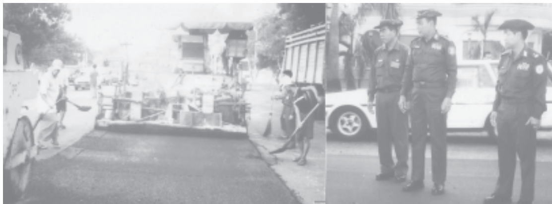
Commander Maj-Gen Myint Swe and Mayor Brig-Gen Aung Thein Lin view tarmacking of Bayintnaung Road.—YANGON COMMAND
