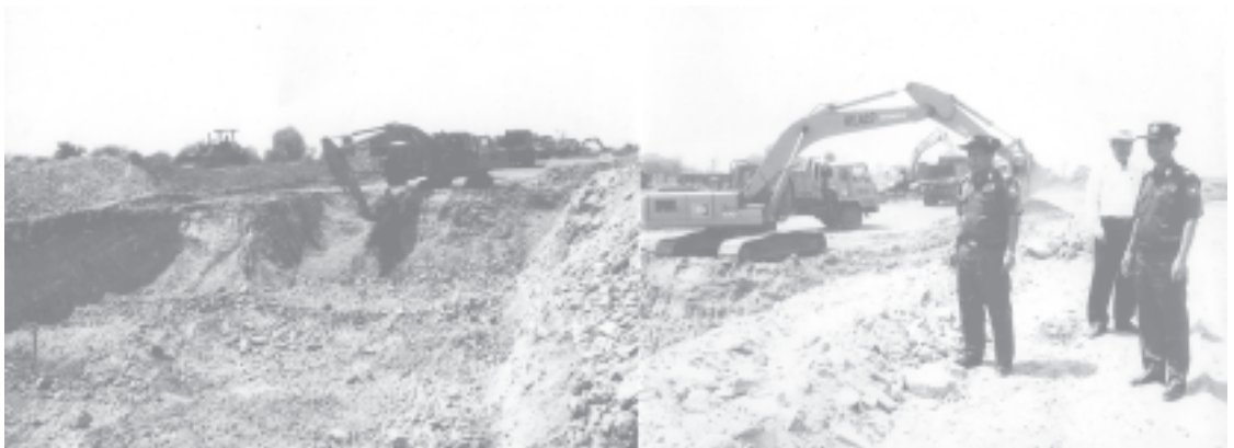
Lt-Gen Ye Myint and party inspect digging of 5400 feet long canal that will link Lunngin and Lethkotpin dams. — MNA
