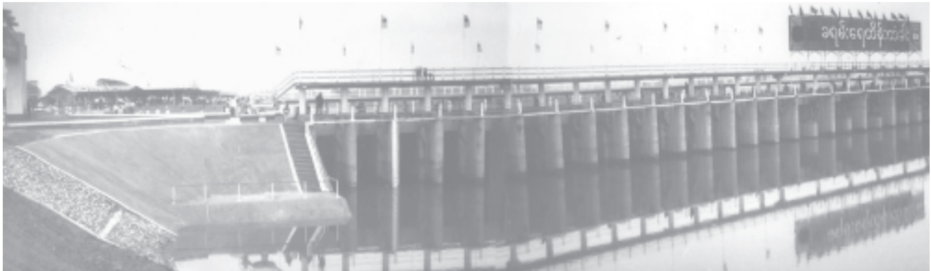
Newly opened Kayan Sluice Gate built on Kayan Creek in Thanlyin Township.— MNA
