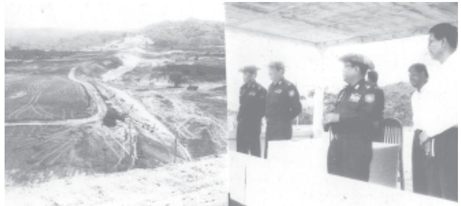
Lt-Gen Maung Bo inspects construction site of Kataik Dam Project in Paung Township.— MNA
