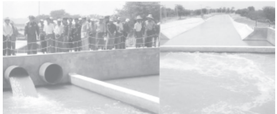
Commander Maj-Gen Ye Myint and Minister for Agriculture and Irrigation Maj-Gen Htay Oo inspect Lawkananda river water pumping project site in Bagan-NyaungU.—AGRI&IRRI
