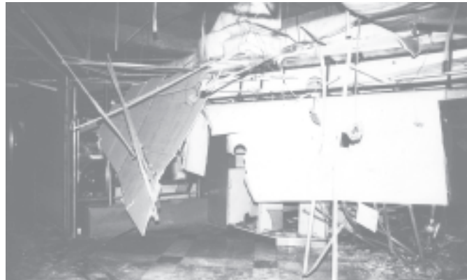
Damages at Dagon Centre in Sangyoung Township after an explosion triggered by a time bomb.— MNA
