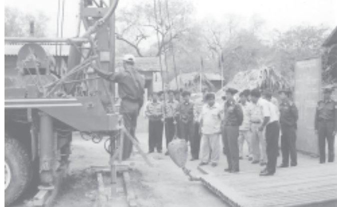
Minister Col Thein Nyunt inspects sinking of tube-well in Oyinywathit in Mya township. — PBANRDA
