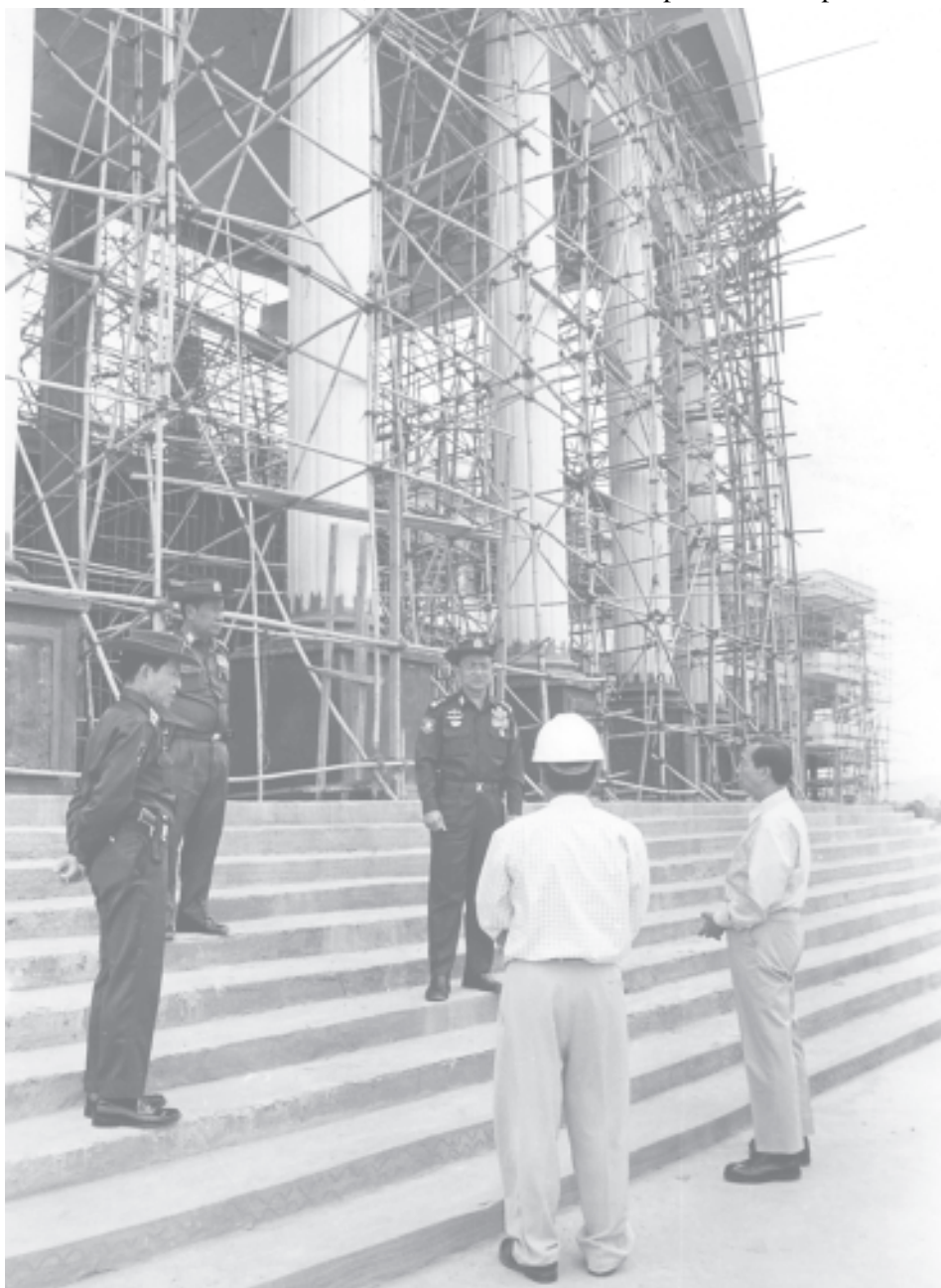
Secretary-1 Lt-Gen Thein Sein inspects construction of Government Technological College in Myitkyina.— MNA
