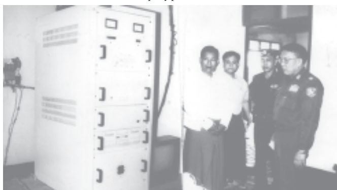
Deputy Minister Brig-Gen Aung Thein inspects TV retransmission station in Tachilek.—MNA
