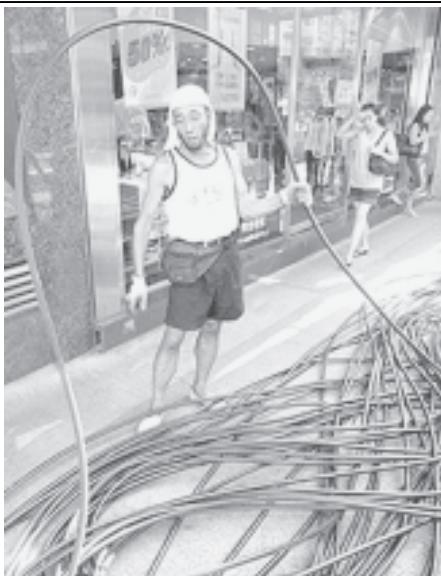
A worker prepares to install telecommunication cables on a street in Hong Kong recently. — INTERNET
