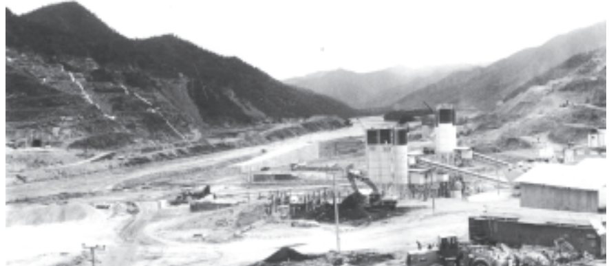
Yeywa Hydel Electric Power Project site to generate 790 megawatts in Mandalay.
