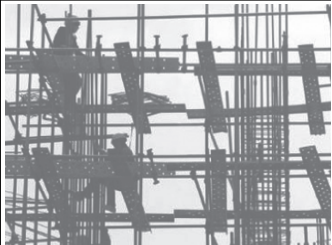
Chinese construction workers erect scaffolding at a construction site in China’s capital Beijing on 20 April, 2005.—INTERNET
