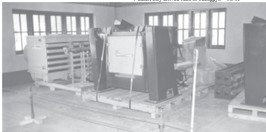
Machinery installed in the foundry plant in Ayethayar Industrial Zone in Taunggyi Township. — MNA
