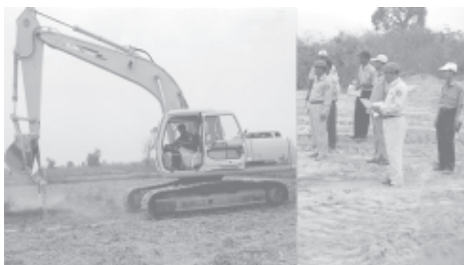
DAD Director-General U Myo Myint inspects construction of the road in Thayawady District with the use of heavy machinery on 4-4-2005.—DAD
