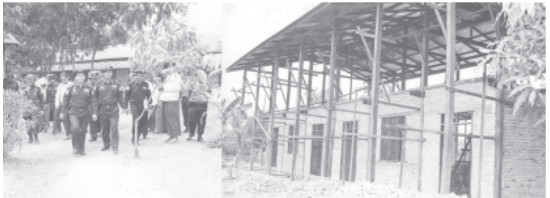
Prime Minister Lt-Gen Soe Win inspects progress in building of extension of school, Paingkyon, Hlaingbwe, Hpa-an District, Kayin State. — MNA
