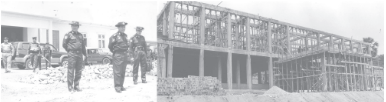
Prime Minister Lt-Gen Soe Win inspects construction of Ye Railway Station.— MNA
