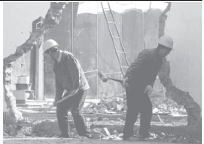
Workers demolish an old brick wall on the construction site of a new office building in Beijing on 2 April 2005 — INTERNET
