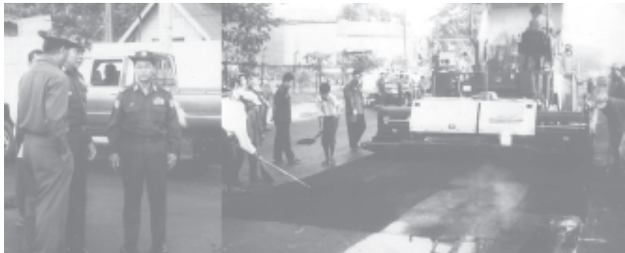
Commander Maj-Gen Myint Swe and Mayor Brig-Gen Aung Thein Lin inspect tarmacking of the road.
