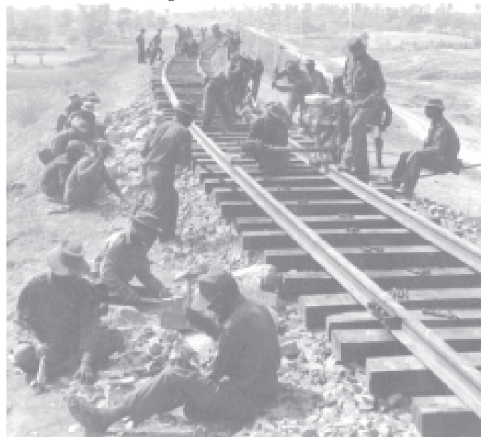
Magway-Taungdwingyi Railroad Project in Taungdwingyi Township, Magway Division, being implemented with the efforts of the Tatmadaw members.
