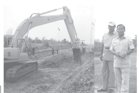
Director-General U Myo Myint inspects progress of district-to-district road in Hmawby.— DAD
