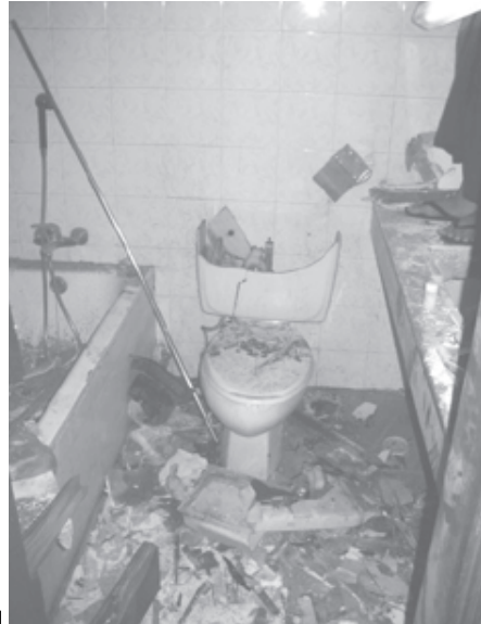
Damages caused by a bomb that went off in the bathroom of PANORAMA Hotel in Kyauktada Township on 19 March. — MNA.
