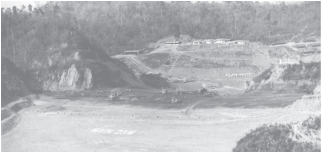
Progress in construction of Khabaung Multipurpose Dam Project in Oktwin Township.— MNA
