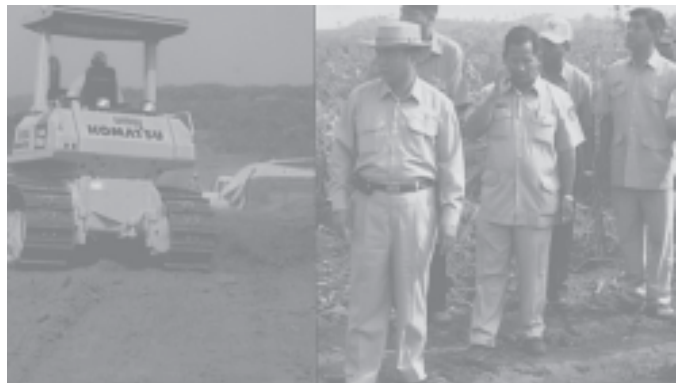
Director-General U Myo Myint of Development Affairs Department inspects construction of the district-to-district road in Hmawby Township.— DAD
