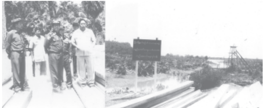
Lt-Gen Maung Bo inspects construction of Payitaung rural bridge on Payitaung Road in Myeik Township. MNA
