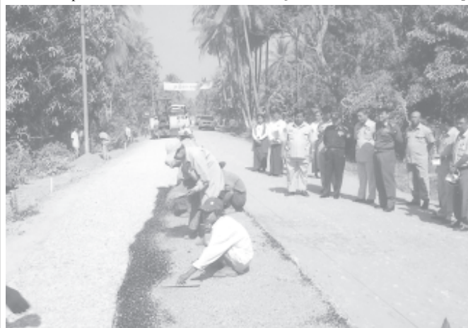
Minister for PBANRDA Col Thein Nyunt inspects repaving of Lanmadaw Road in Kyaiklat Township on 28-2-2005.— PBANRDA
