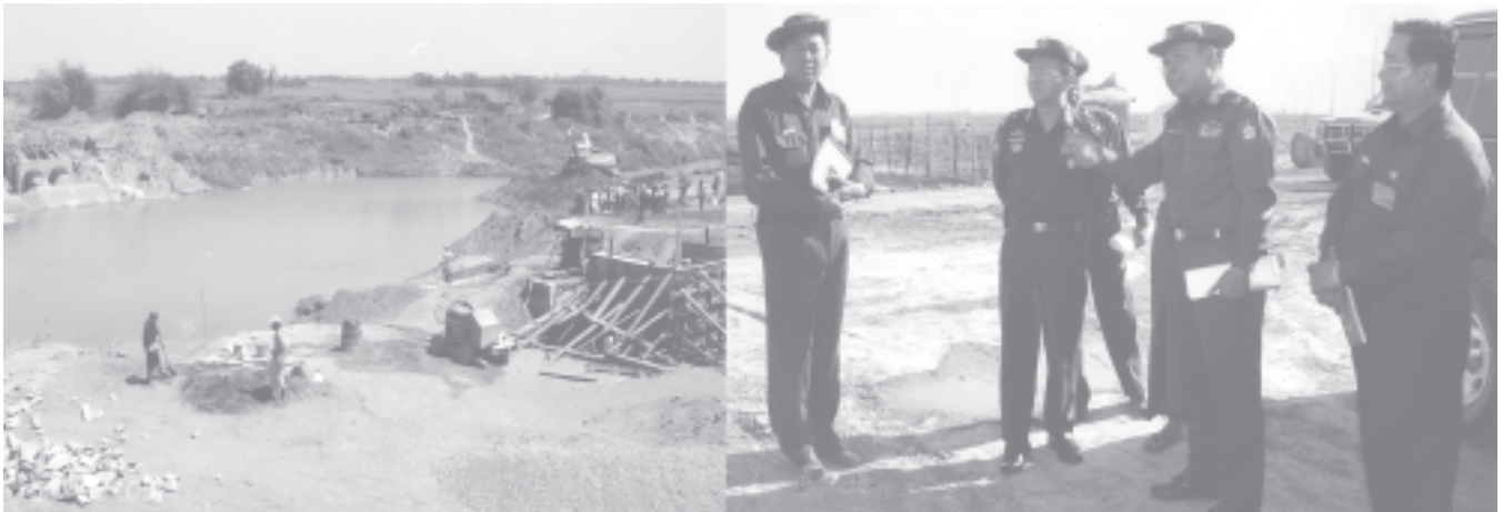
Secretary-1 of the State Peace and Development Council Lt-Gen Thein Sein inspects construction of syphon crossing Ngamoeyeik Creek near Kalihtaw Village (West) in Hlegu Township.— YCDC
