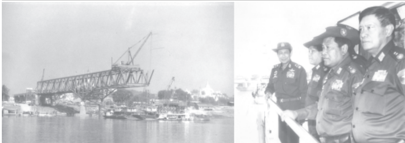
Vice-Senior General Maung Aye inspects installation of steel beam between RP 7 and RP 8 of Ayeyawady Bridge (Yadanabon). — MNA
