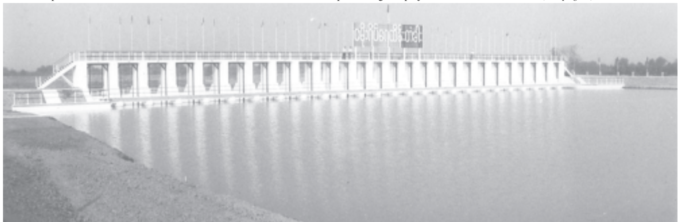
Newly-opened Ngamoeyeik Sluice Gate with 26 valves seen after opening ceremony.— MNA
