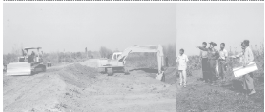
Minister Col Thein Nyunt inspects construction of the road linking Kya-in Village and No 3 Highway in Hmawby Township. — DAD
