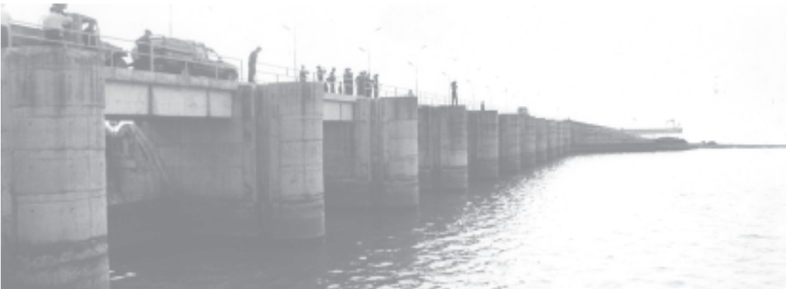
The spillway of Thaphanseik Dam built near Thaphanseik Village in Kyunhla Township.—MNA
