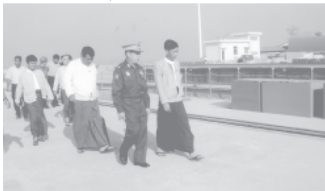
Minister for Transport Maj-Gen Thein Swe inspects construction of 12,000-ton-capacity dry dock of Myanma Shipyards.—TRANSPORT
