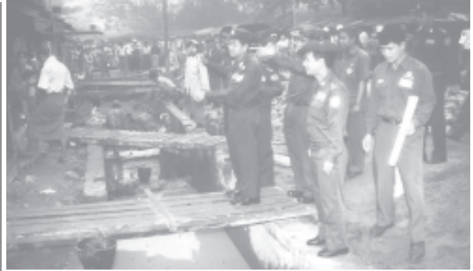
Commander Maj-Gen Myint Swe inspects construction of concrete drain in U San Pe Ward of Thingangyun Township on 19-2-2005.
