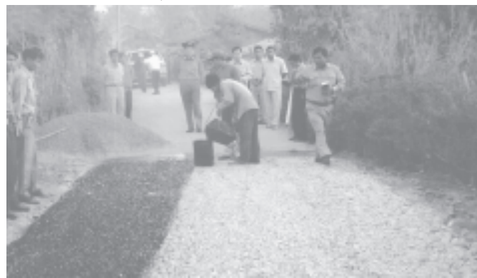
Minister for PBANRDA Col Thein Nyunt inspects repaving Myitta Road in Kengtung Township on 9-2-2005. — PBANRDA
