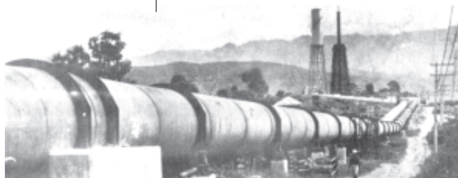
A pipeline of Bilu Creek Hydel Power Plant in Kayah State.
