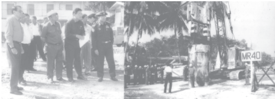
Minister for Construction Maj-Gen Saw Tun oversees driving of MR 40 bored pile for the railroad of Thanlwin Bridge (Mawlamyine) on Mawlamyine Bank.— CONSTRUCTION
