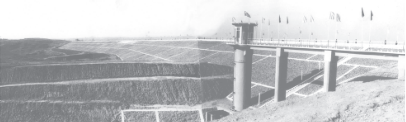
Pade Dam on the Pade Creek in Aunglan Township, Thayet District, Mangway Division.—MNA
