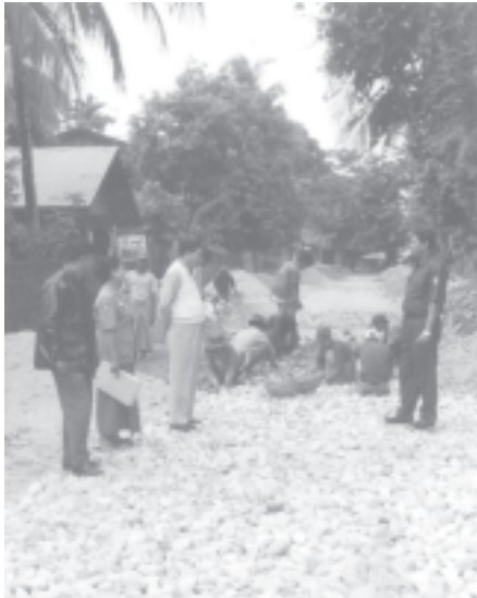
Officials of Waingmaw Township Development Affairs Committee oversee construction of a rural gravel road.—KYEMON
