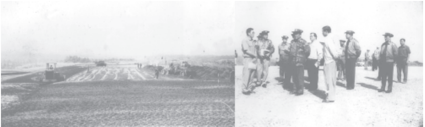
Lt-Gen Ye Myint inspects progress of Hkamti airport runway extension project in Sagaing Division. —MNA
