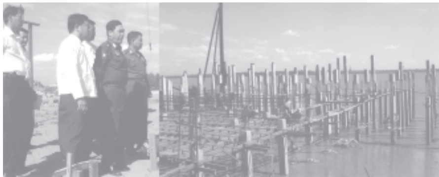
Ministers Maj-Gen Thein Swe and Brig-Gen Maung Maung Thein inspect progress in constructing Tharkayta wharf. — TRANSPORT
