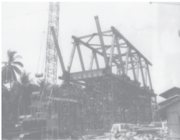
Minister for Construction Maj-Gen Saw Tun inspects installation of iron frames at Pyapon Bridge. —CONSTRUCTION
