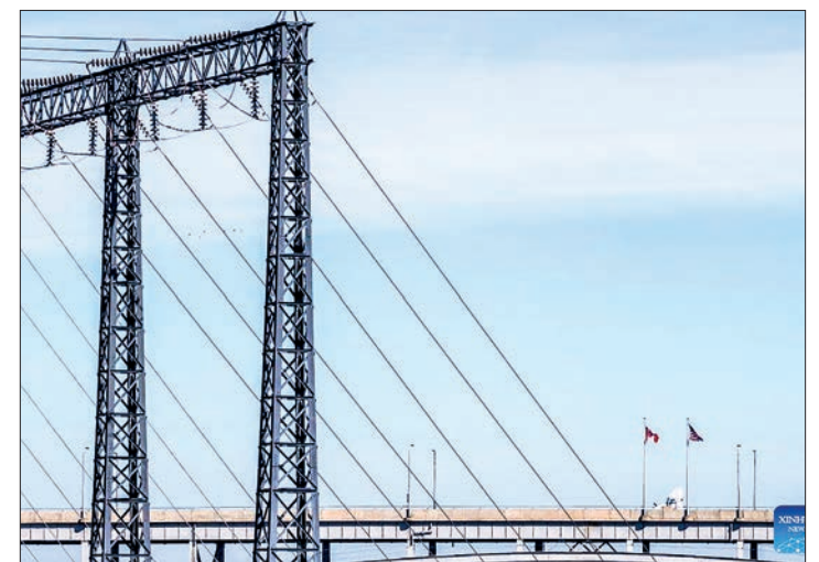
Photo taken on 10 March 2025 shows power lines leading from Sir Adam Beck Generating Stations of Canada in Niagara Falls, Ontario, Canada. Canada’s Ontario government on Monday officially applied a 25 per cent surcharge on all electricity exports to three US states. PHOTO: XINHUA
