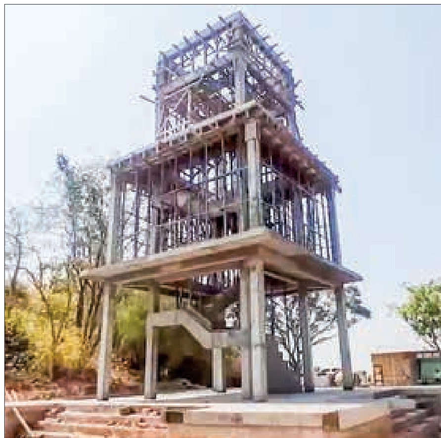
This photo shows a viewing tower in the ancient city of Sri Ksetra under construction.
