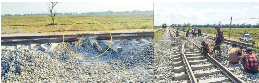
Photos show mine blast damage and railway repairs.
