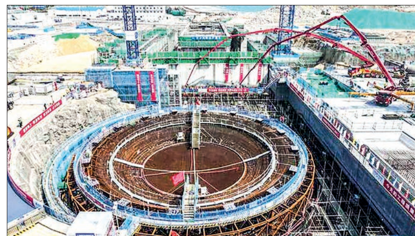
A total of six reactors have been planned for the project. PHOTO: CGN
