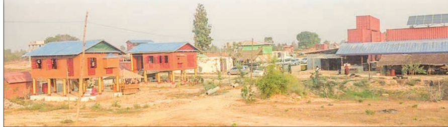
This photo showcases a Buddha Garden and a volunteer relief village being built near milepost 203 on the Yangon-Mandalay Expressway.
