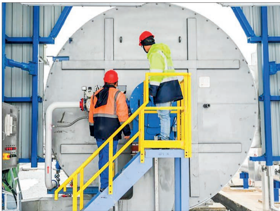
Chinese employees check the ground station facilities of the Tuz Lake underground natural gas storage expansion project, in Aksaray province, Türkiye, 12 February 2025. PHOTO: XINHUA
