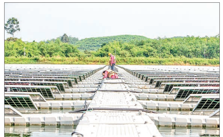
Staff members check the cable of the solar floating project in Rayong, Thailand, 11 April 2022. PHOTO: WANG TENG/XINHUA/FILE
