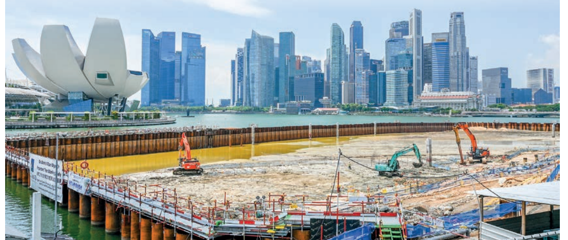
Excavators are seen at a construction site with the city’s skyline in the background in Singapore on 23 October 2024. PHOTO: AFP
