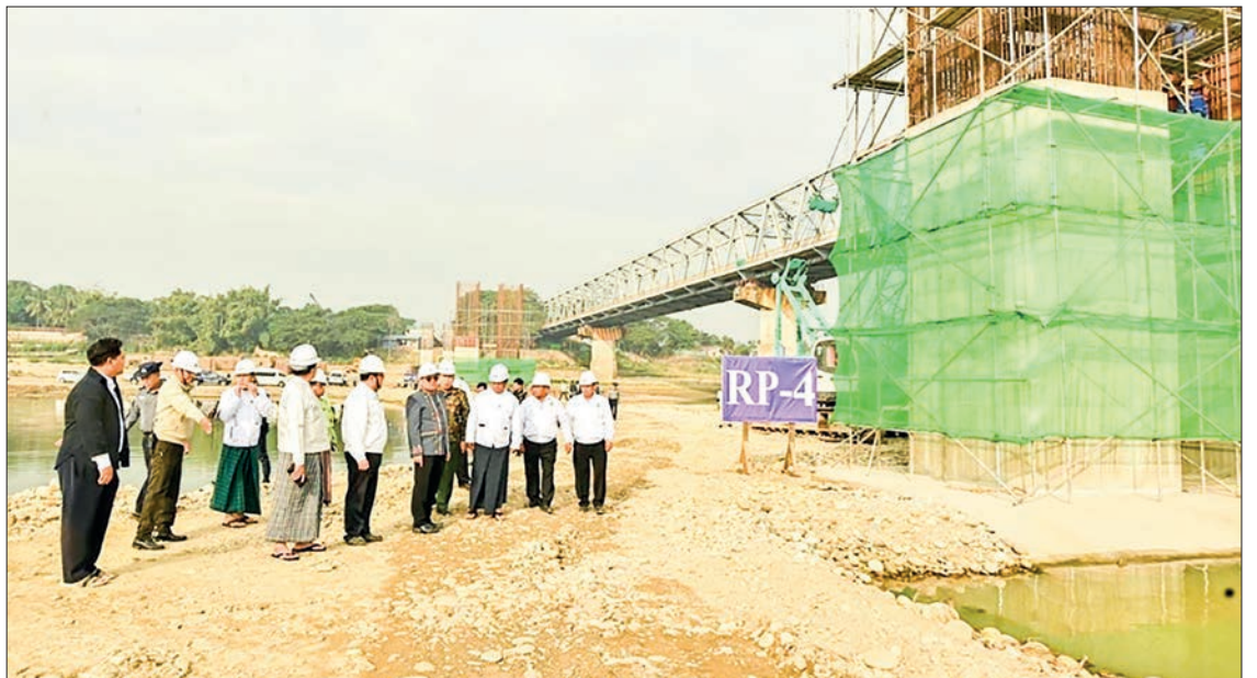
This photo shows officials inspecting the construction site of the Bala Min Htin Bridge II.
