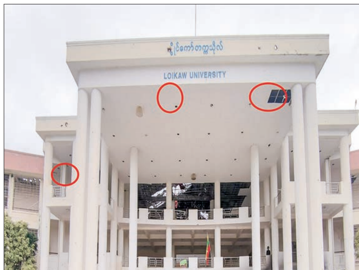
One of the damaged buildings at Loikaw University.
