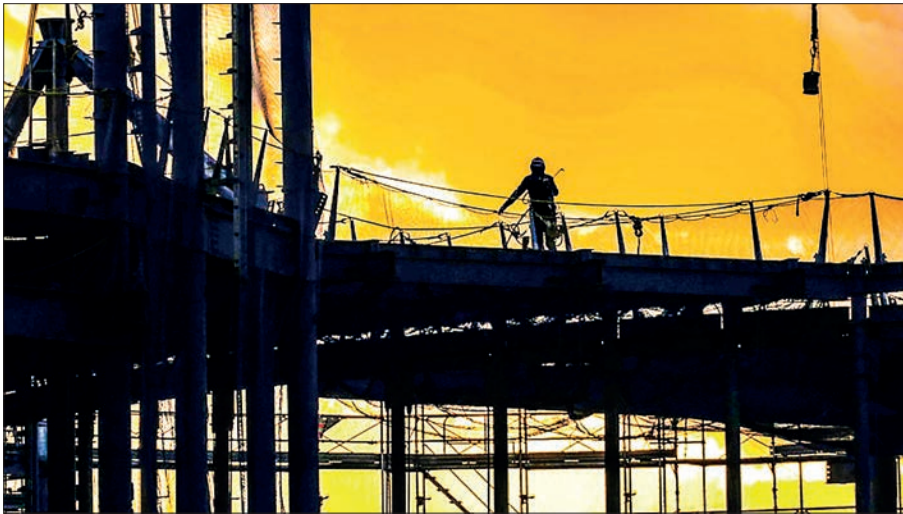
File photo taken in Osaka in November 2023 shows a construction site on Yumeshima, a man-made island in Osaka Bay. PHOTO: KYODO
