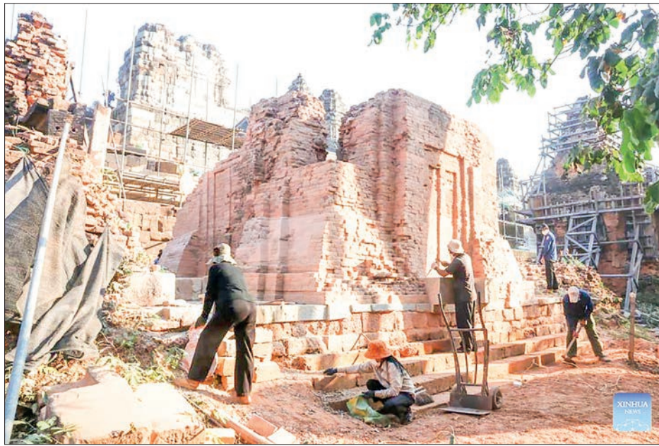
This undated photo shows staff members working at the restoration site of Tower 15 at Phnom Bakheng temple in Siem Reap province, Cambodia. Archaeologists of Cambodia's APSARA National Authority (ANA) have completed the restoration of Tower 15 at Phnom Bakheng temple in the Angkor Archaeological Park in northwest Siem Reap province, said an ANA's news release on Monday. PHOTO: XINHUA
