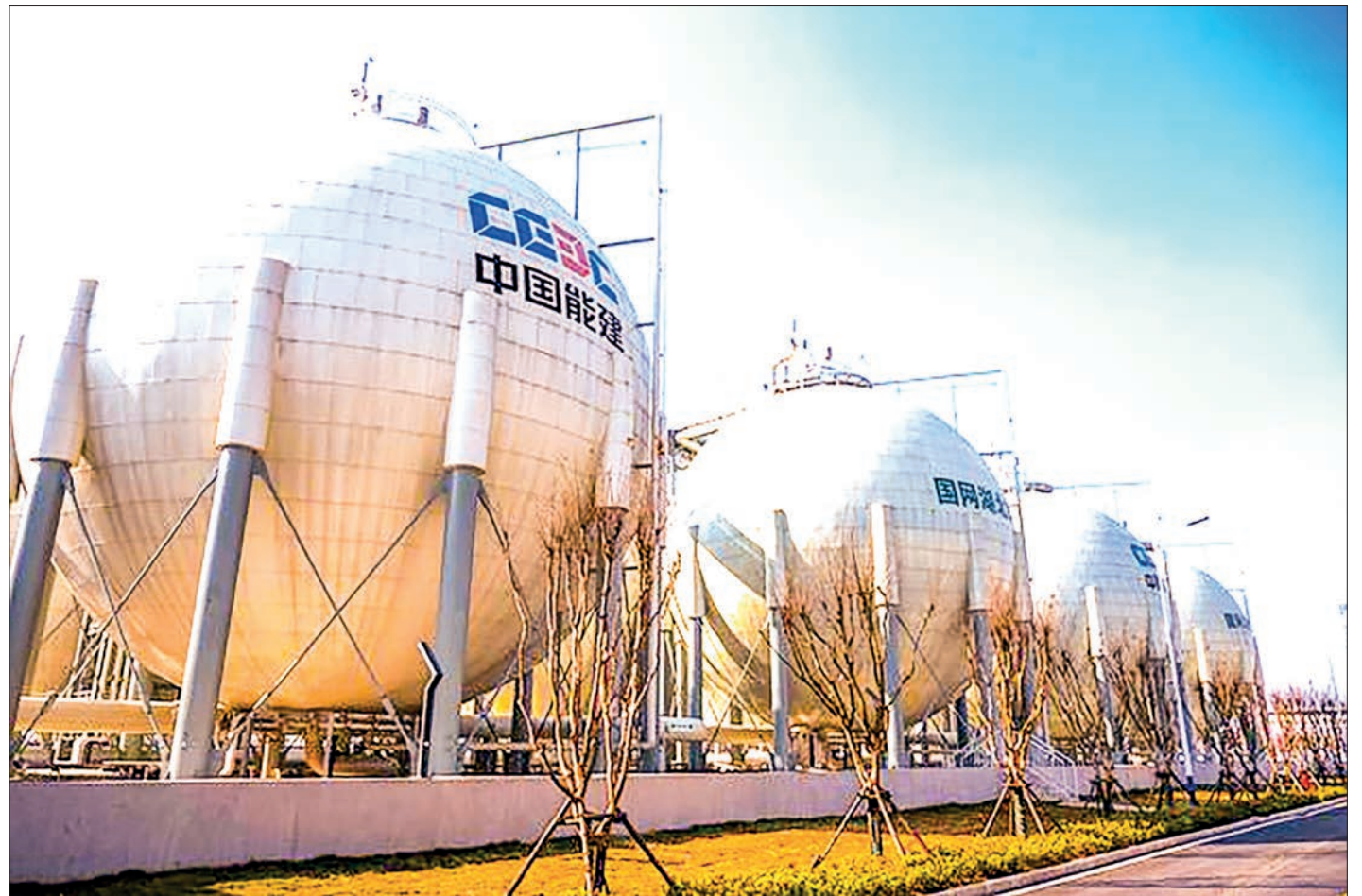
This photo shows a corner of the 300 MW compressed air energy storage station in Yingcheng City, central China's Hubei Province, 24 December 2024. PHOTO: XINHUA
