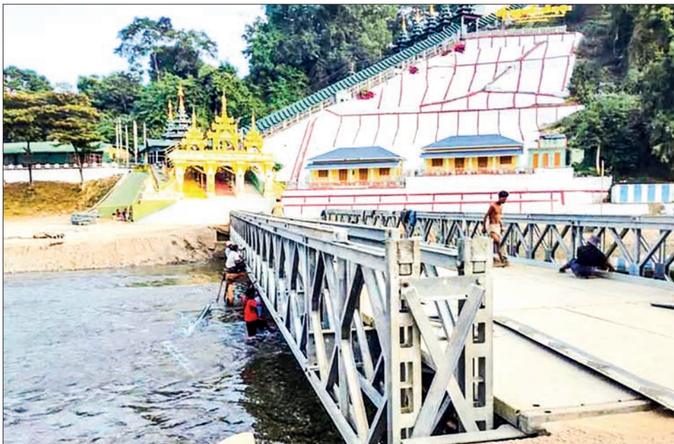
This photo showcases the steel Bailey bridge being installed to provide pilgrims access to the lower golden footprint of the Mann Shwesettaw Pagoda.
